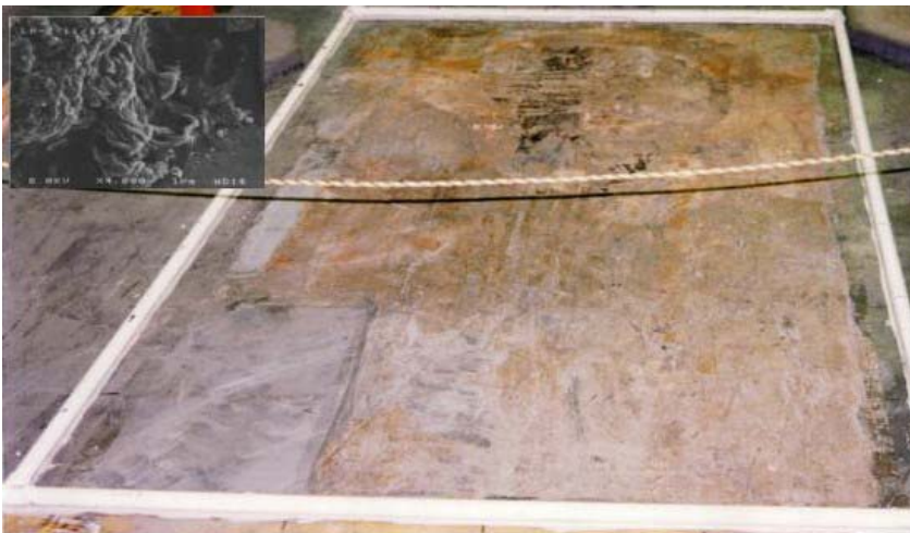
Fig. 3. Loosened surface material on concrete. Inset: Microscopic image of degraded surface material.
